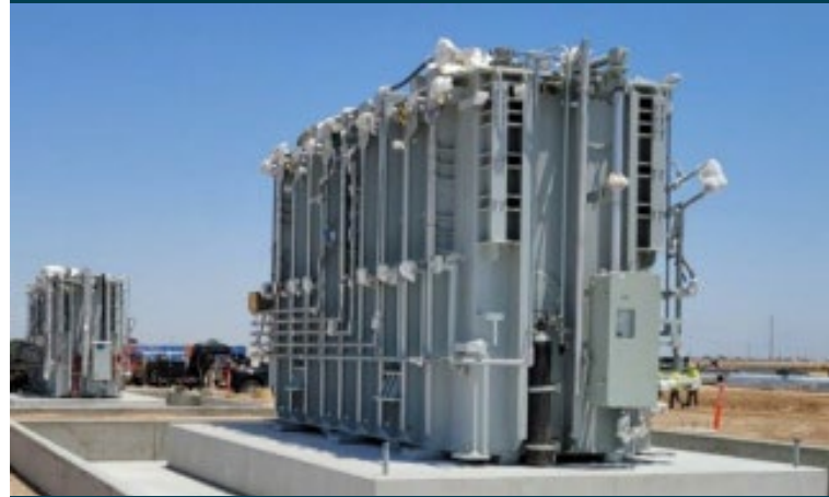
Big Rock: 200 MW asset with 100 MW of RA deliverability
