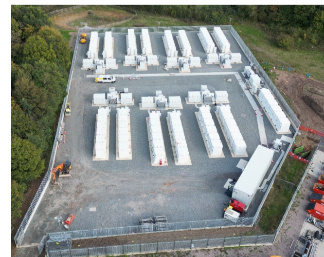
Enderby (57 MW / 57 MWh)
